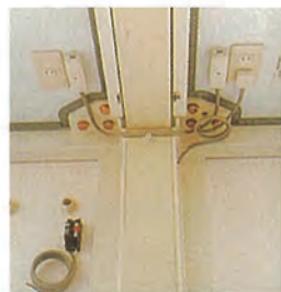
連棟部入電側
