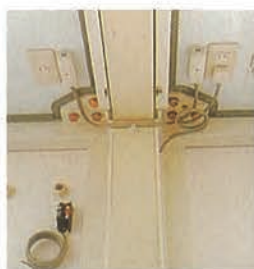
連棟部入電側
