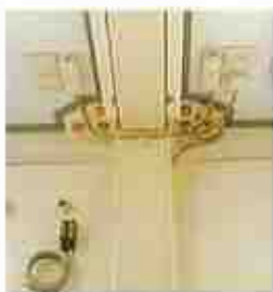
連棟部入電側
