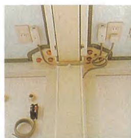
連棟部入電側
